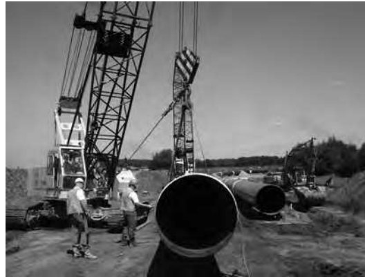
Figure 2.1. A pipe with a diameter of 1.2 m. (Source: Open Grid Europe GmbH (OGE).)
